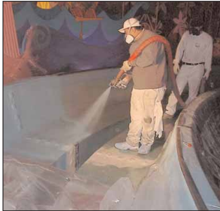
A crew member applies polyurea on the water course of one of the park's rides using Graco's Reactor proportioner and Fusion spray gun.
